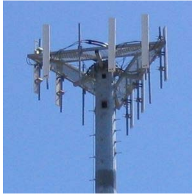
Figure 2-7. Typical Cellular Base Station Tower
