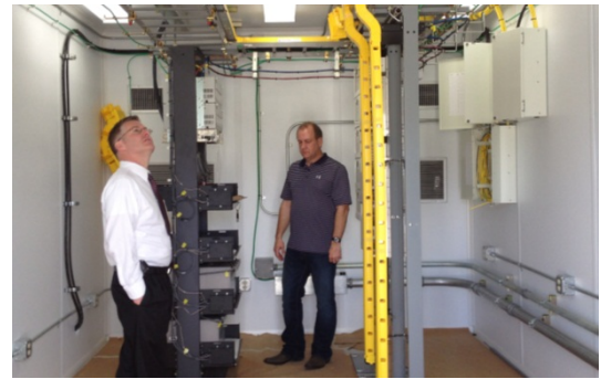
A NTIA Federal Program Officer visits a Sho-Me MO Middle Mile Project equipment shelter in Jefferson City, Mo.
