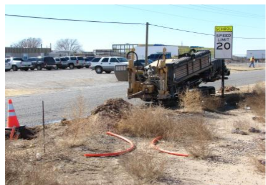
ENMR crews drill a hole to install fiber at the project's second market site.
