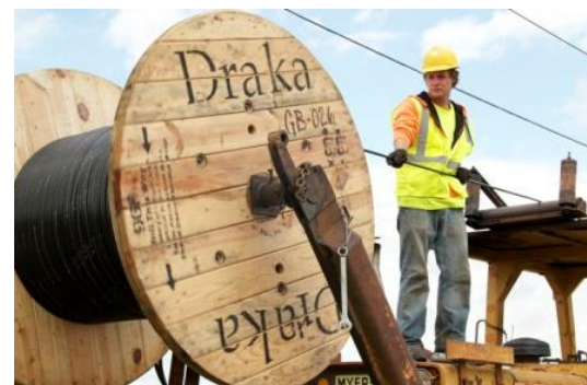
A Com Net crew member helps lay new fiber-optic cable lines in rural Ohio.
