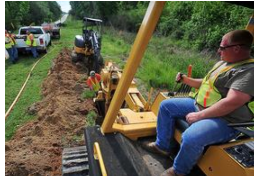
Workers for Troy Cablevision dig a trench to install a broadband cable in Ozark, Ala. The project has connected 49 community anchor institutions through June 2012.
