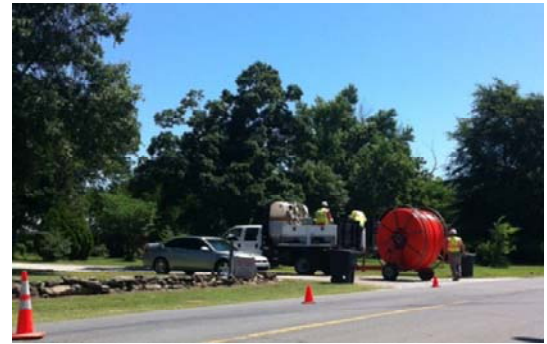
A construction crew in Warner, Okla., deploys new fiber that will bring broadband service to Connors State College.
