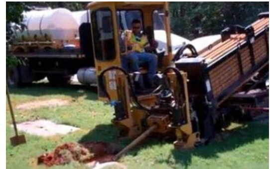
A member of Maryland DoIT drills a site in La Plata, Md., to deploy fiber as part of the One Maryland Broadband Network project.
