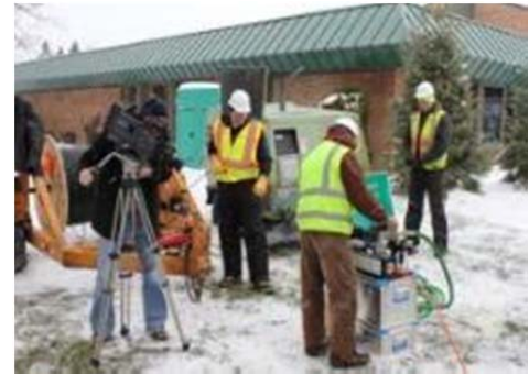
Merit Network construction crew members feed fiber into the conduit at the project's groundbreaking ceremony in Manistee, Michigan.
