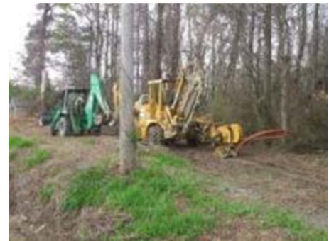
A plowing and trenching crew installs fiber along a route that runs from Rocky Mount to Greenville, North Carolina.
